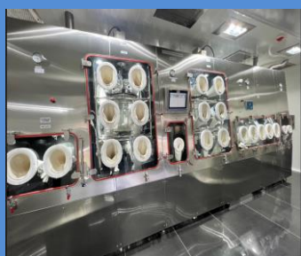
Isolator with Reactors, PNF, VTD & Powder processing
