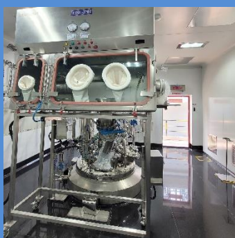
Reactor with Charging Isolator
