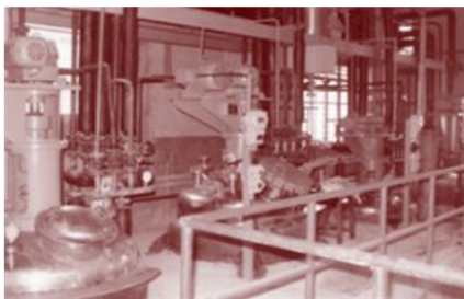
Triton opened its second manufacturing facility at Jeedimetla to produce multiple APIs
